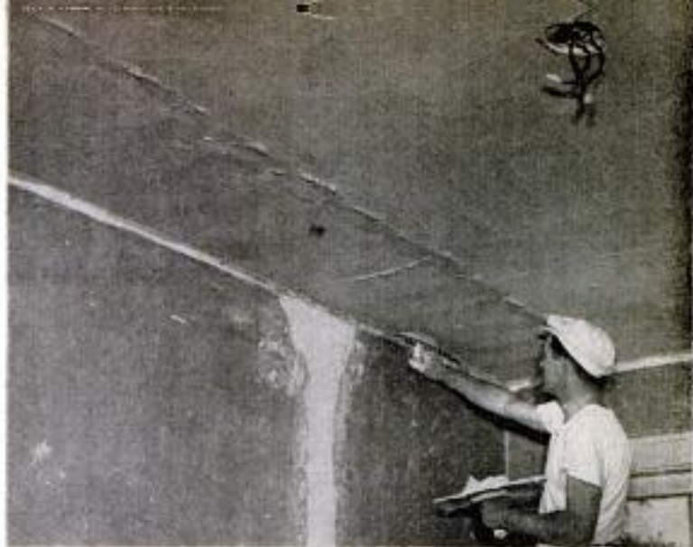
Last of base coat is being troweled on ceiling. Note above how plaster is troweled toward center of room. Light weight of ready-mixed plaster makes job easy
